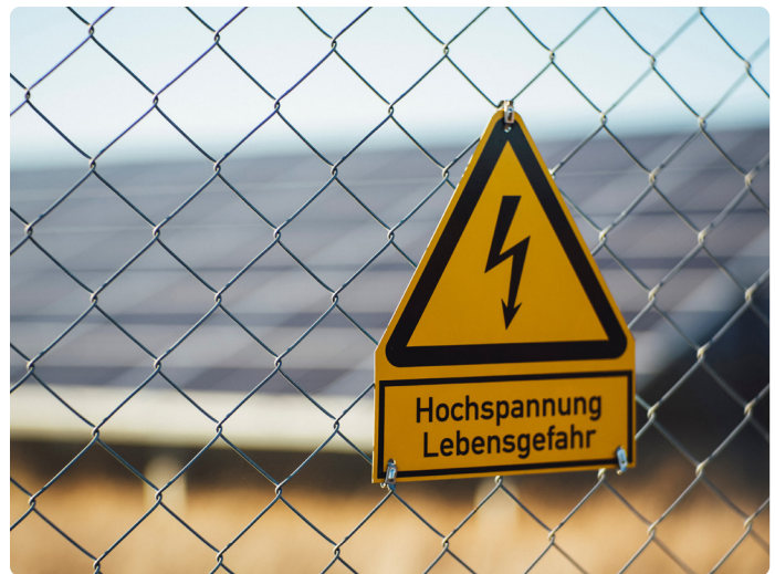
All solutions have their challenges. A sign warns of high voltage at a German electricity installation.
