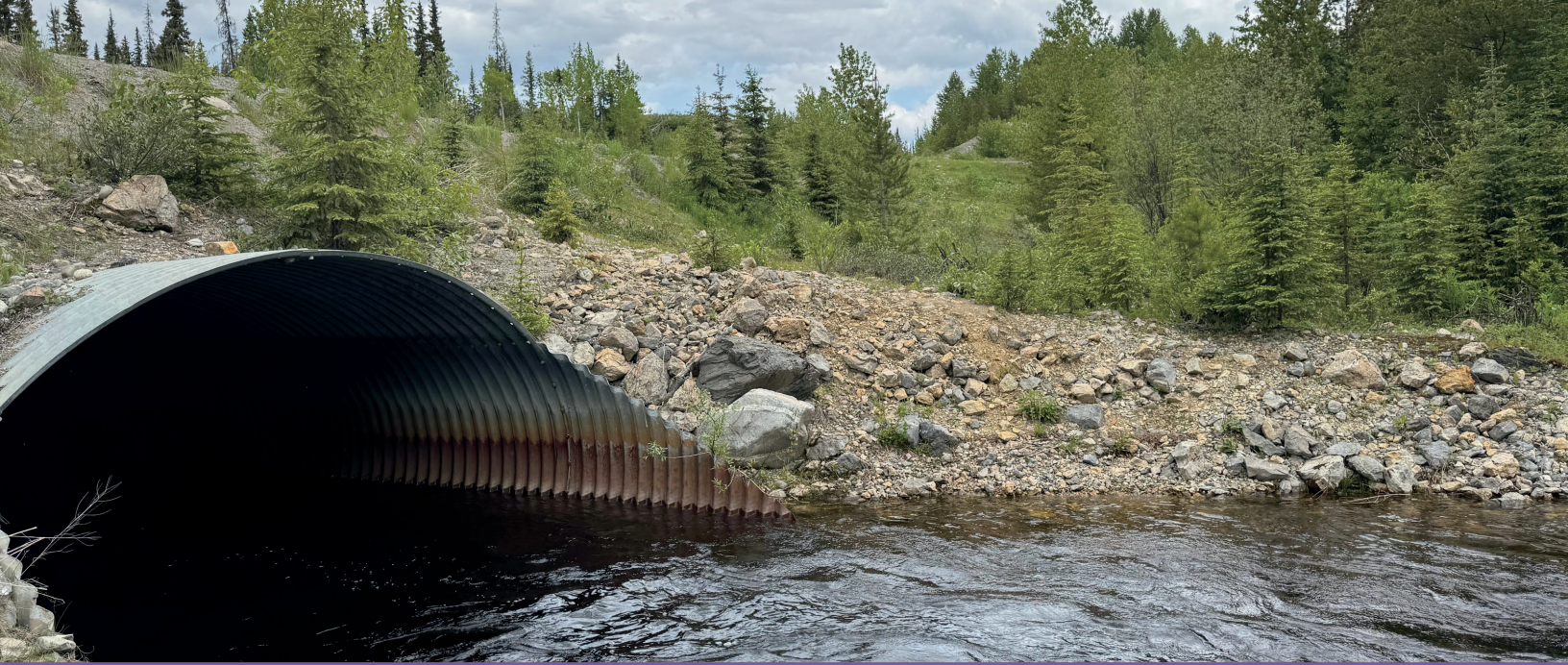
Figure 5. Stream crossings and drainage structures play an important role in how water moves through forested watersheds and can influence both road stability and aquatic habitat.
