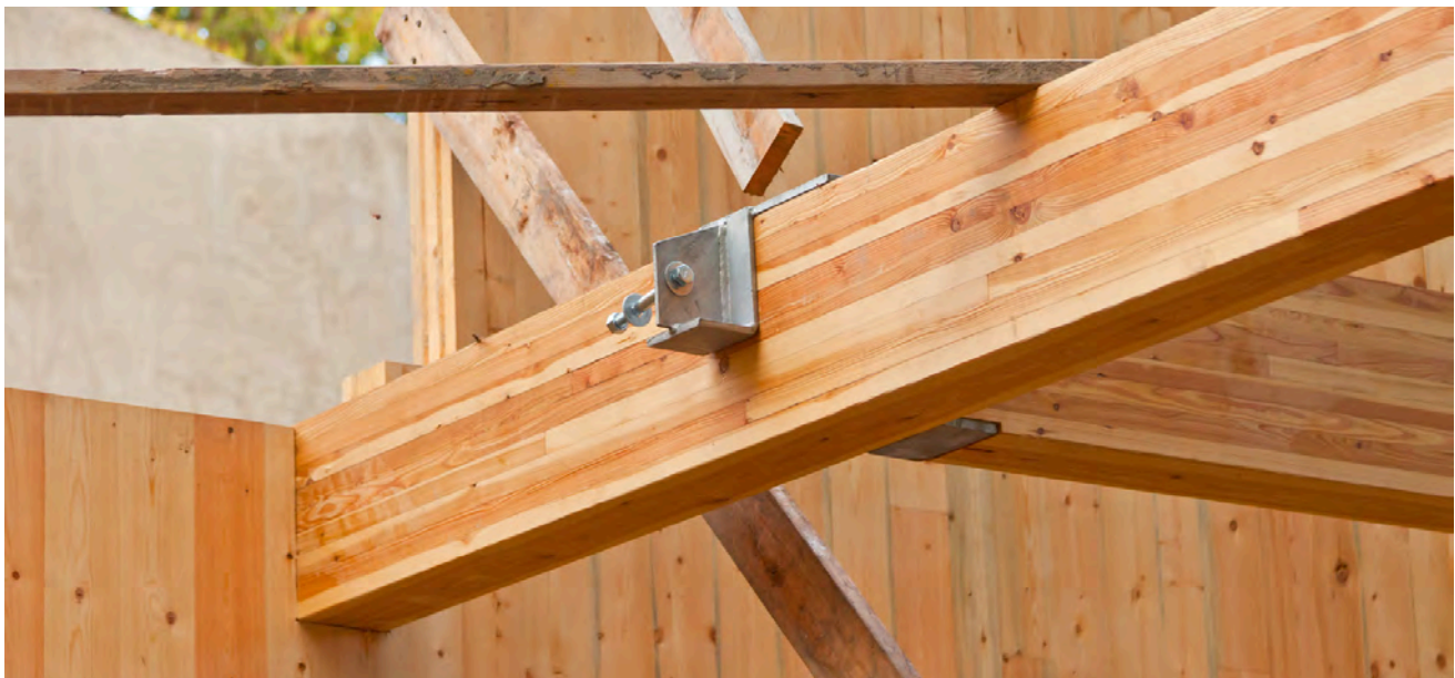
Bioenergy Research & Demonstration Facility at UBC. Photo Credit: KK Law, courtesy naturallywood.com
